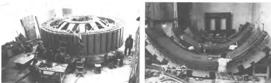
Figure 7 Manufacture of stator and rotor of 24 MVA, 10 kV, 125 r.p.m. synchronous generator for Mariborski otok HPP (1946)
