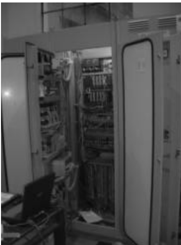
Fig. 5. PLC with turbine Governor GU 2
