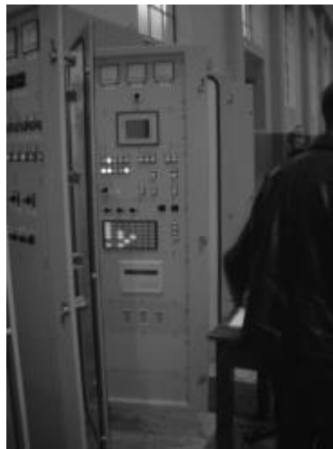
Fig. 6. Control Cubicle of GU 2
